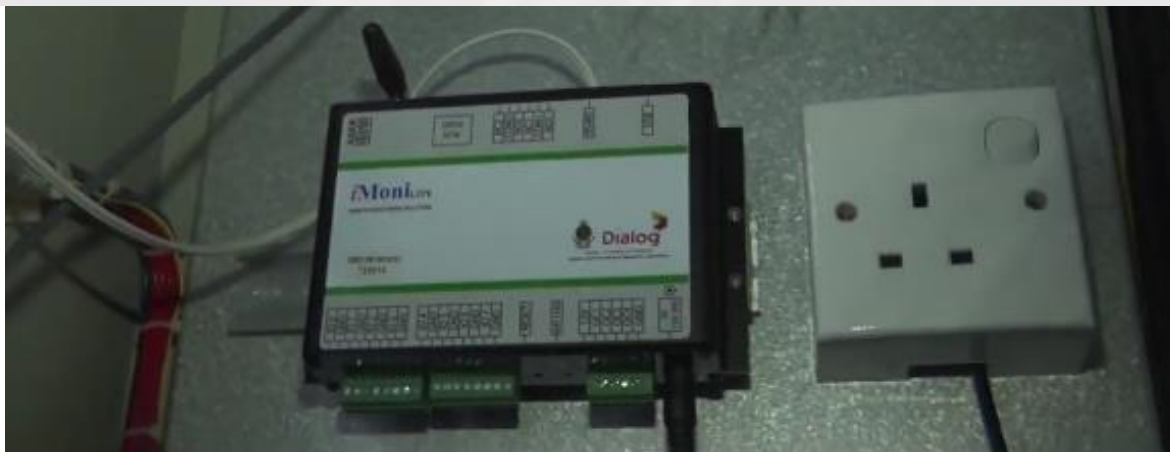
Remote Telemetry Solutions for base station & ATM monitoring
